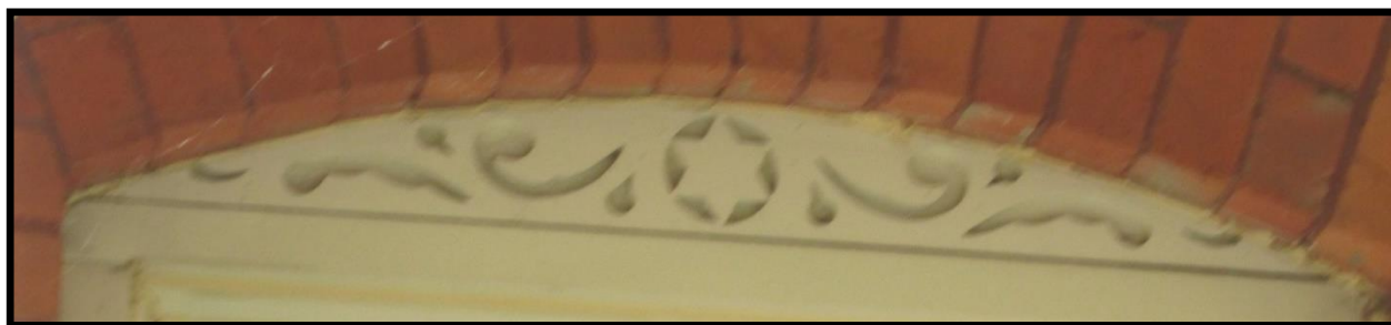
Figure 2.1: The 6-pointed star in the lintel of the doorway to 261 Clarence St. The same patterns are also on the lintels of all of the windows and doorways. Photo by Katherine Lipsett.
