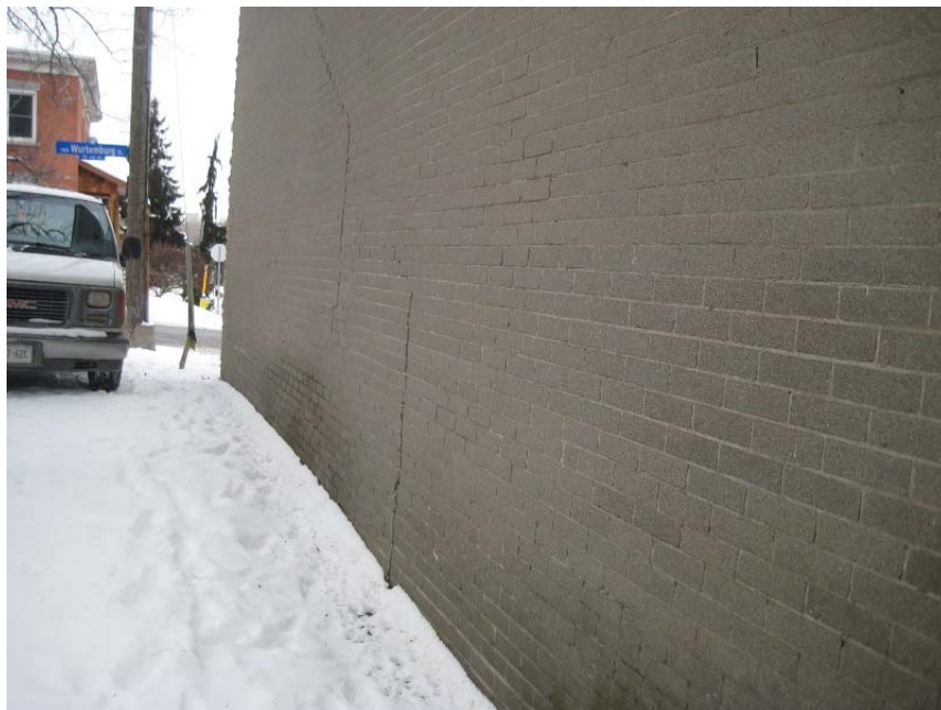
Photograph 10: View looking west towards the south-facing exterior wall showing further structural damage. This photograph also shows a utility pole with what is thought to be a source of electricity to the Site (hydro wires). There were no pole-mounted transformers observed on the Site or nearby.
