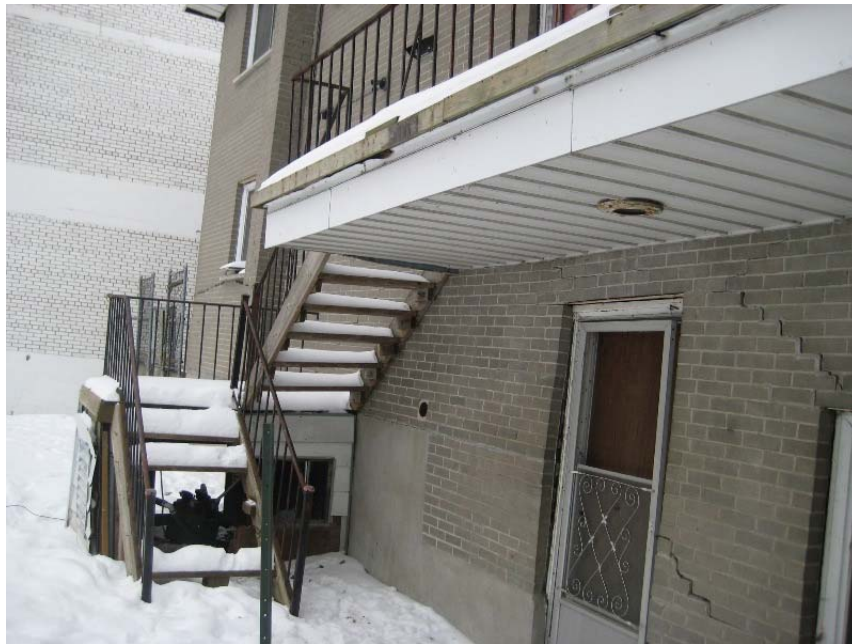
Photograph 7: View looking south towards the east-facing exterior building wall, showing structural damage to the stairs and foundation (visible cracks).
