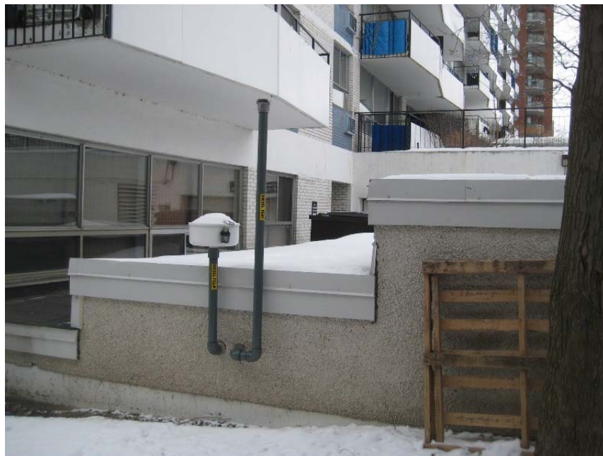
Photograph 6: View looking south towards the vent and fill pipes associated with the apartment buildings. It is interpreted that these pipes connect to an aboveground storage tank in the parking garage, which is used to fuel a backup generator. These pipes are located approximately 10 m away from the property.
