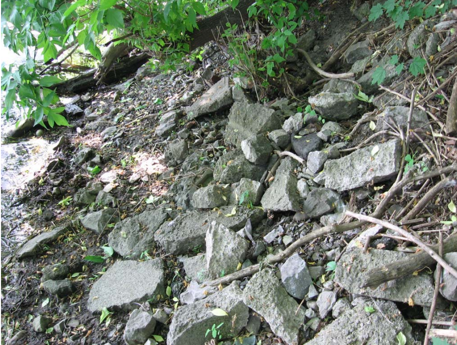
Photo 12. Shoreline showing broken concrete that has been moving downslope toward the river – May 25, 2010.
