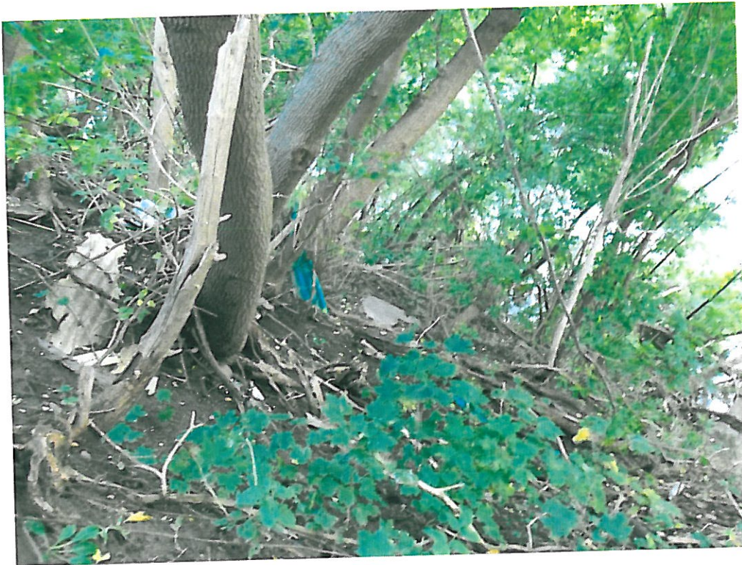
Photo 7. Close-up of fill on slope, and lack of vegetation at grade
