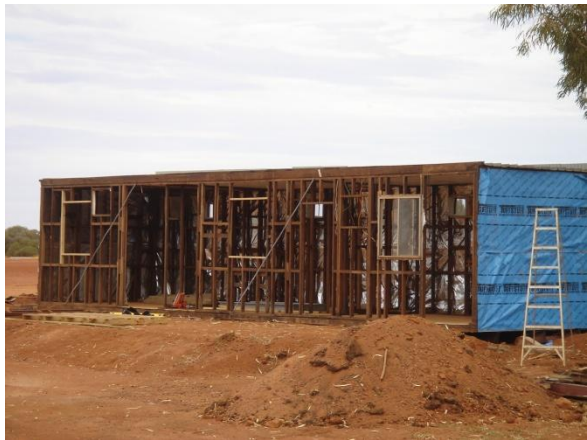
The Old Laundry Donga is being refurbished into the new Motel Units.
