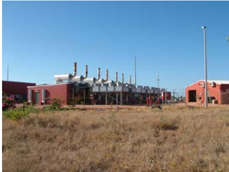
Exmouth Gas Fired Power Station
