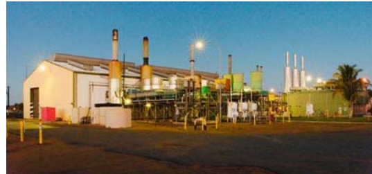
Carnarvon Power Station is the only Power Station in Regional WA that can run on diesel fuel or a combination of Diesel and Gas
