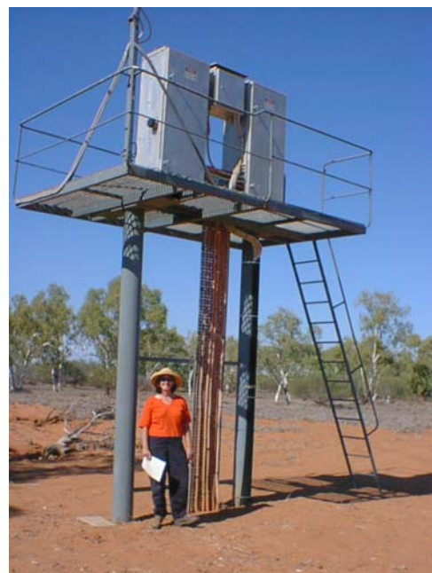
Remote controlled electrical switchboard for four bores in bore field. Note: the platform is 1m above flood level
