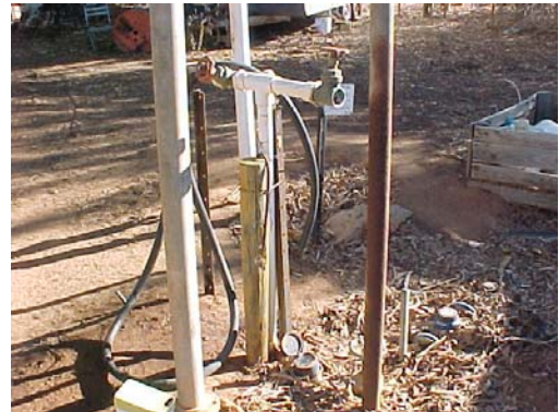
This tee piece is used to fill poison tanks for spraying. It rises from the same pipe work that leads to the house tank.
