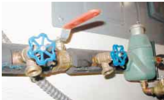
Three valves make up the drain/fill assembly.
